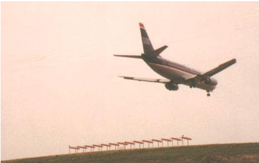
Localizer antenna array for instrument landing system.
