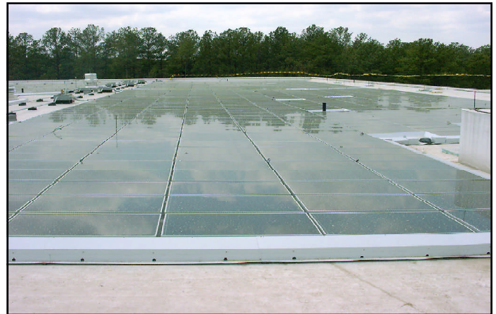
Figure 2: Commercial PV system at EPA facility in Research Triangle Park, NC.
