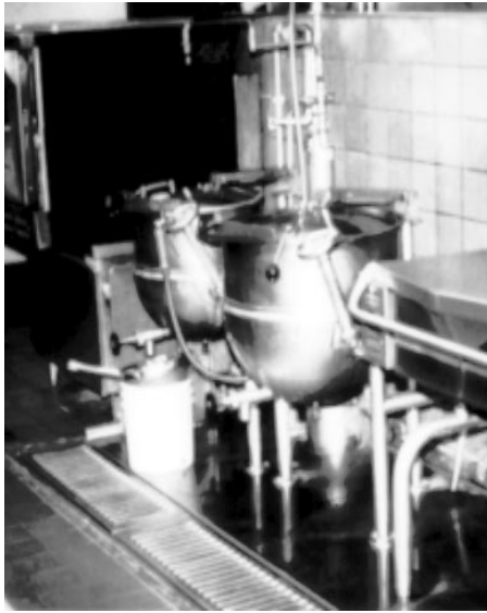
Fig. 5. Area under food preparation equipment is raised above a smooth stainless steel floor, allowing for easy cleaning of food spills and open to prevent harborage.
