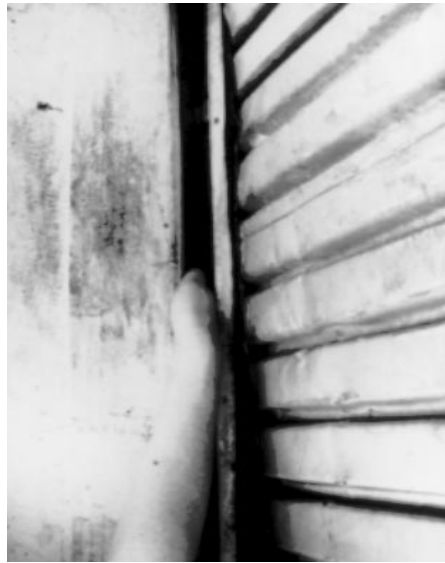
Fig. 8. Large gap between roll-up warehouse door frame and wall, allowing for easy rodent access.
