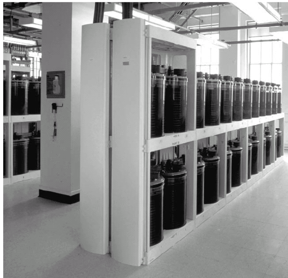
Round Cell Batteries at this central office switching station will be in service for several decades, assuming water is added once every ten years.
